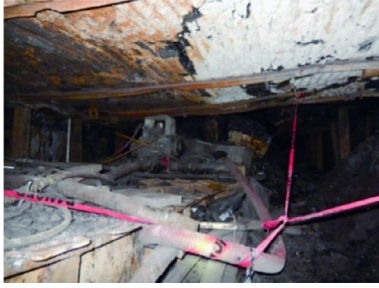
Fig. 4. Roof condition outby the second roof fall in the belt entry.
