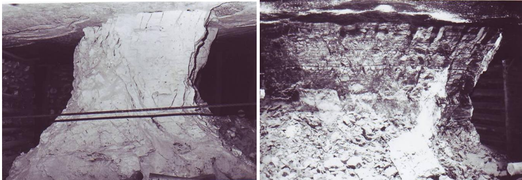
Fig. 5.2.8 Failure of pillars due to fault (left) and joints (right) (Mokgokong and Peng, 1991)
