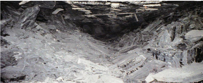
Fig. 5.6.3 Typical pillar collapse. Both ribs sloughed off severely, followed by moderate skin falls. The debris piles from both ribs met at the entry center (Peng, 2007)
