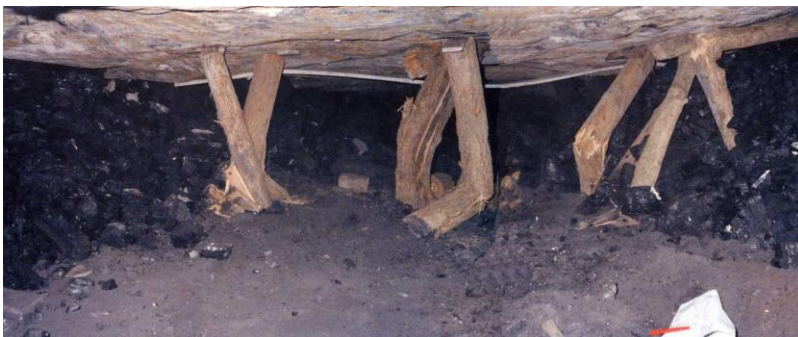
B. Cross sectional view of pillar failure
