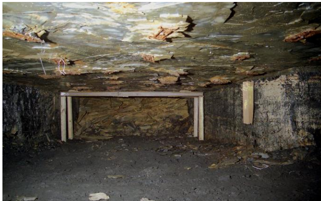
Fig. 5.10.1 Flooding caused the immediate roof to peel off between bolts, while the pillar remained intact. A large roof fall occurred in the background (Peng, 2007)
