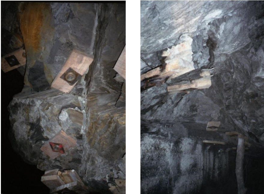
Fig. 8.5.2 Cracks in the upper seam roof that were caused by lower seam mining had been sealed with calcite (white) (left), a typical roof fall in the upper seam (right) (Peng, 2007)
