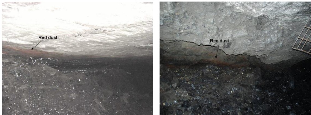
Fig. 9.3.1 Red dust at the roof of the bump sites (see color photos in Appendix 3)
