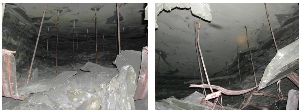
Fig. 10.5.4 An example of a roof fall (two scenes) due to weathering of weak roof (Peng, 2007)
