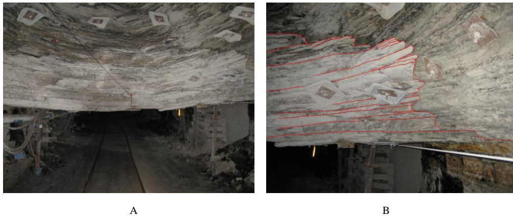
Fig. 10.2.2 Entry fall: A, inby wall of the roof cavity, and B, beam structures of the right edge of the roof cavity shown in A (Peng, 2007)
