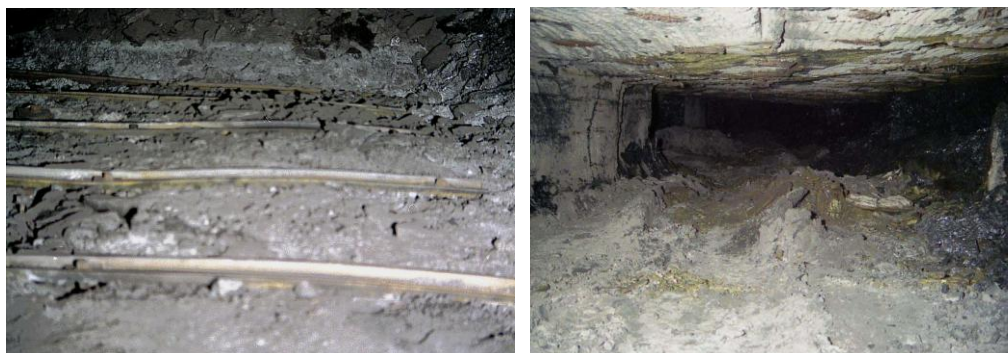
Fig. 10.6.5 Comparison of floor condition between floor-bolted and non-bolted entries (Peng, 2007)
