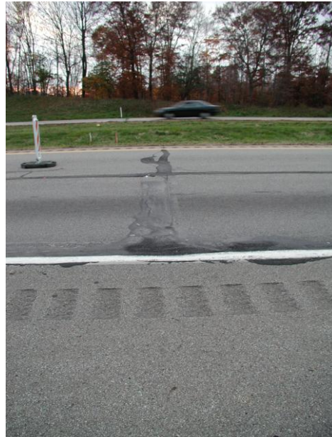
Fig. 13.11.2 Bump on an interstate highway formed over the central portion of a longwall panel
