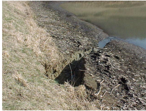
Fig. 13.11.1 Ground crack formed over a longwall panel
