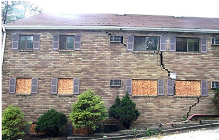
Fig. 13.11.3 Step cracks on the basement wall of a residential house
