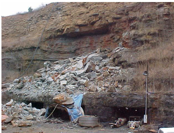
Fig. 14.4.2 Wedge type of slope/highwall failure. Note that portals below the failed block in bottom photo
